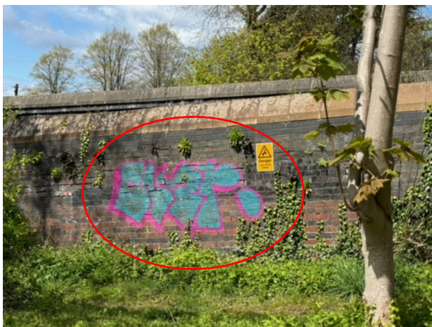
ON WALL IN CAR PARK OFF REDDICROFT, OPPOSITE REAR OF VESEY HOUSE
